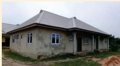
Twin 2-Bedroom Flats Under Construction by BCT Staff and subvention from Goodnews BC, Lagos.
